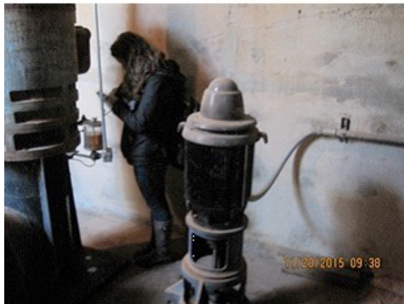
(c) 20-hp 1000-gpm pump
